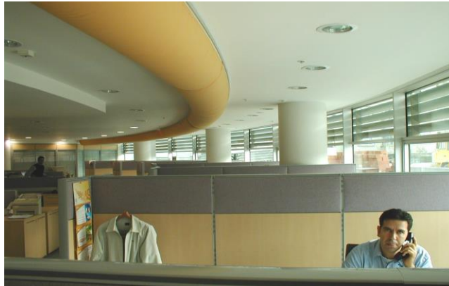
A low impulse textile duct terminal in exposed installation
