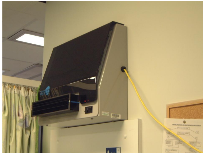
Ionisers in use in a UK Hospital
